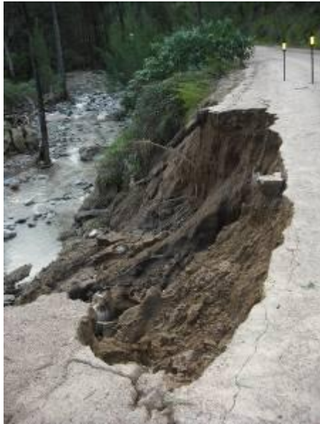
Photo 3: Roadside soil erosion caused by floods (Photo: Malcolm Donnelly)
