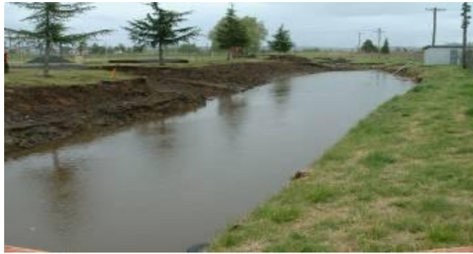
Photo _: A collection barrier being constructed at the rear of the soccer fields
