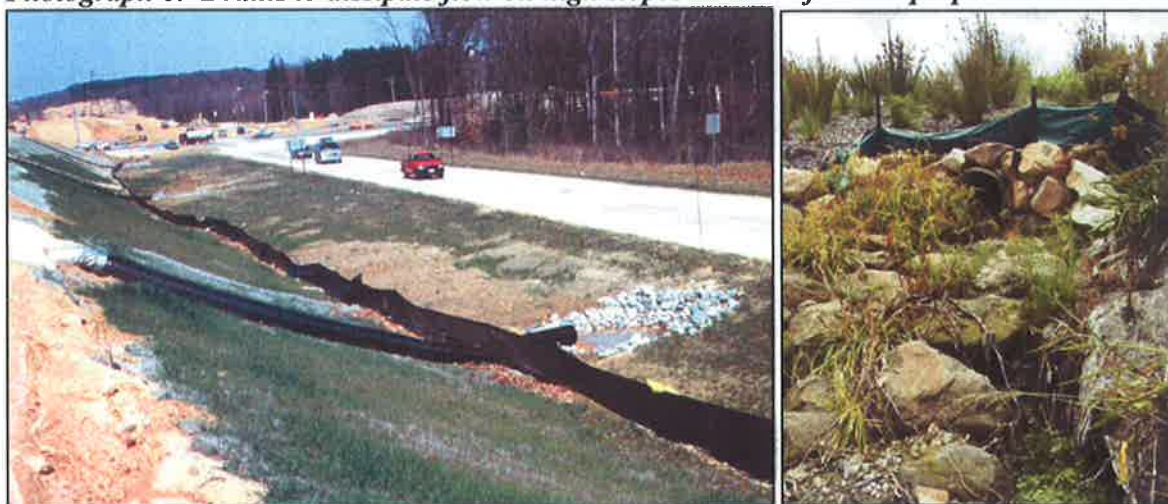
Photograph 6: Drains to dissipate flow on high slopes – HDPE flex & riprap chute drain
