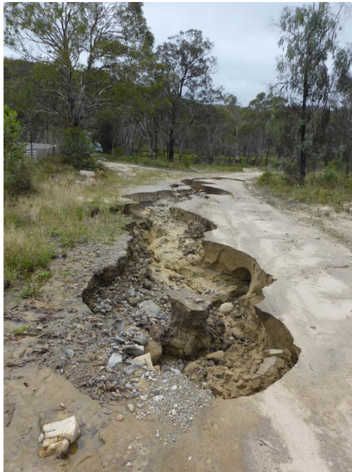
Image 2: Flood Damage on Sara River Road
