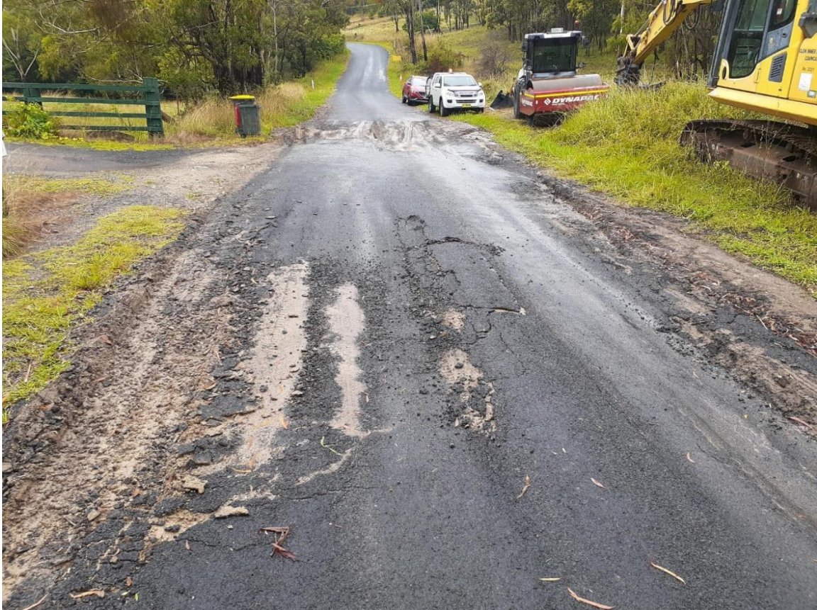
Image 1 – Damage on Blue Hills Road
