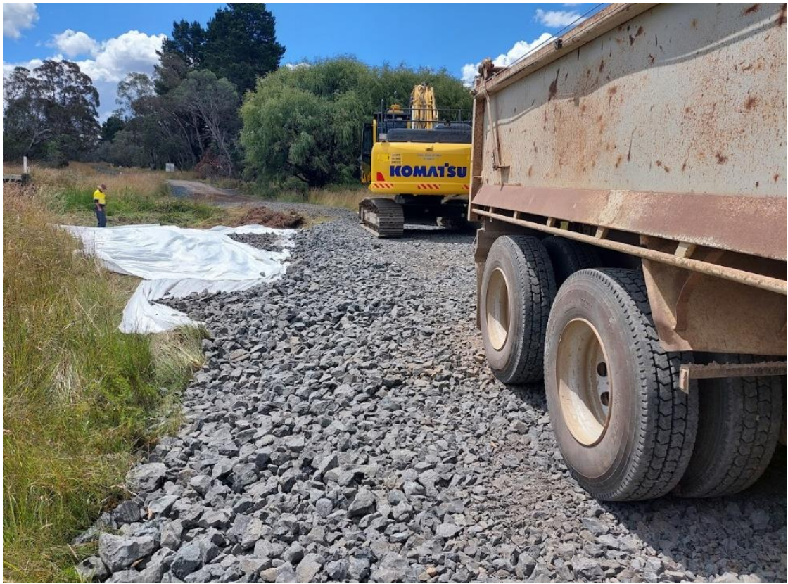
Image 6: Construction of the side access track across Yarrow Creek at the Mt Mitchell Road bridge site
