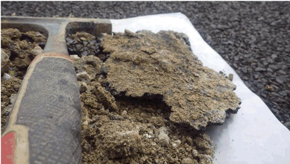
BH09 - Poor bituminous seal to granular base course bond
