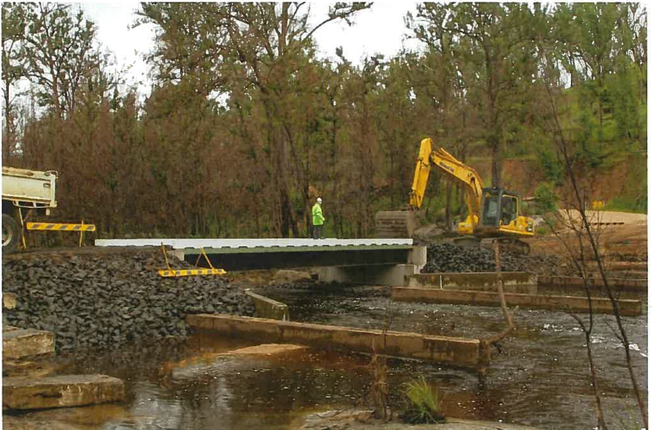
Image 1: Emergency side track installation after Wytaliba bridge was lost through natural disaster (fire)
