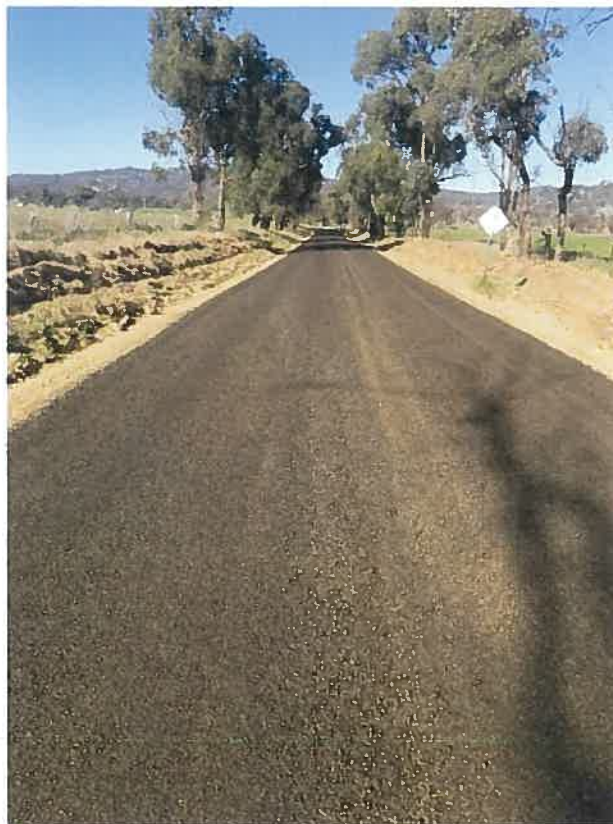
Image 2: Graded Aggregate Seal on Yarraford Road
